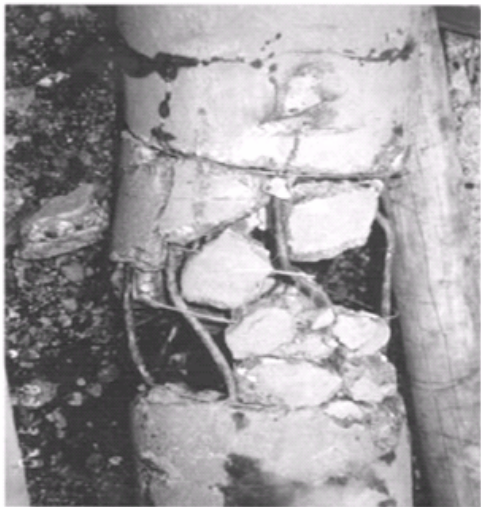
Fig. 17. Damage to pile by 2m of lateral ground displacement during 1964 Niigata earthquake (Yosuda et al.1999)
