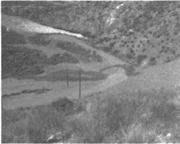
Figure 10. Area A completed. Flow along toe of surcharge berm is from observation well OB-8 which became artesian with high reservoir elevation and a small seep in the abutment rock.
