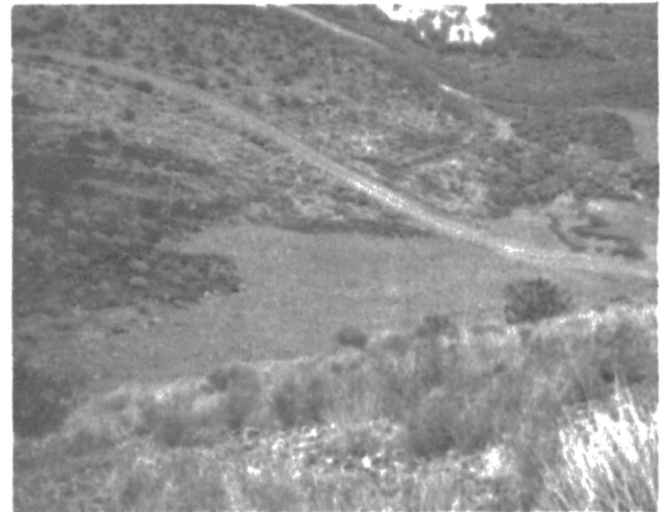
Figure 11. Area B completed. Damp spot in center is from seepage exiting through fractures in the bedrock.
