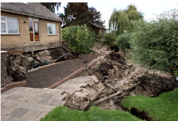
Fig. 6. Circular slip surface failure of the south-quay
