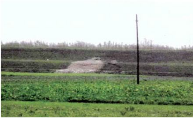
Fig. 1. Water flow through the upper part of the Serchio river embankment at Nodica during the December 2009 flood (Autorità di Bacino Fiume Serchio, 2010).
