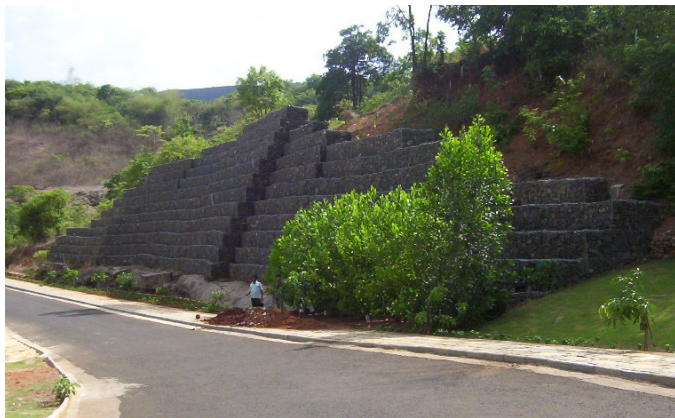
Fig.10 Gabion wall along roadside in AVSLC project.
