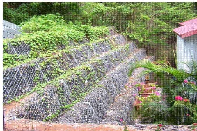
Fig.13 Gabion walls perfectly integrated with flora, AVSLC project.
