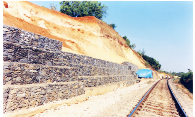
Fig.3 Gabion toe wall for Rockfall protection along Konkan Railway route
