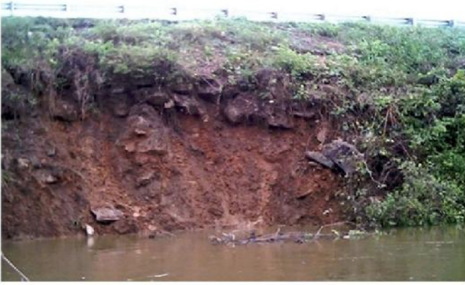
Fig. 3. Photograph taken on 10/11/2002 of slide on 10/10/2002. Note pre-existing rip rap covering the slope and that the slide progressed up the slope by the end of the day
