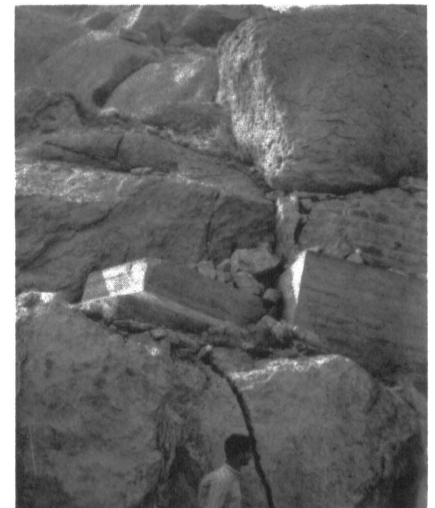
Fig.9 The earthquake fault of the Sefid-Rud dam and its induced rockfalls.
