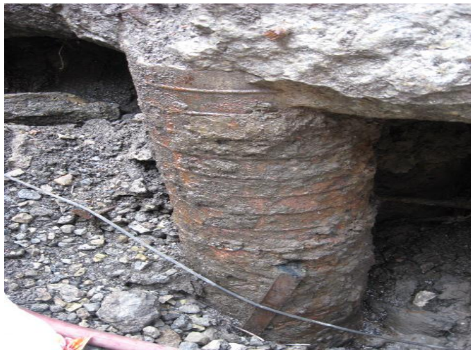
Fig.9. Exposed Pile Showing Thin Steel Casing
