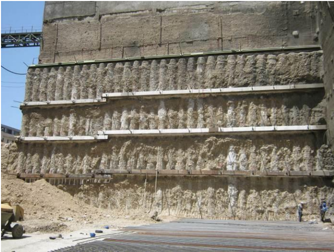
Fig. 14. A view from eastern side of the tower; at this point, excavation is complete and the construction of the foundation of the intended building has begun
