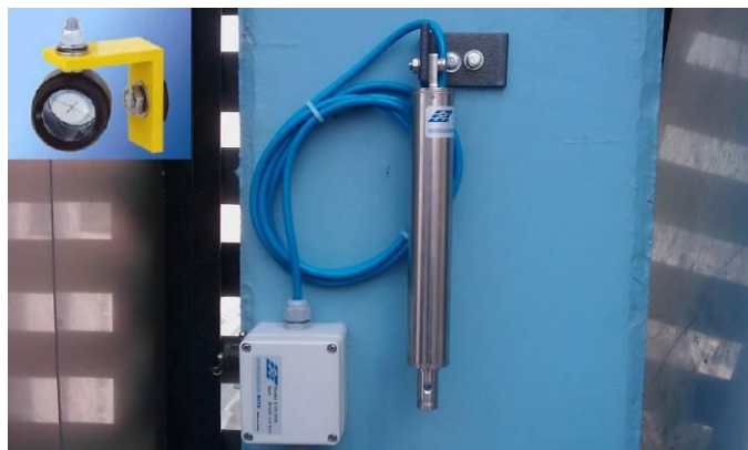
Fig. 17. Tilt meter number 01 on the tower rooftop and a sample of the mini prism targets used in the project
