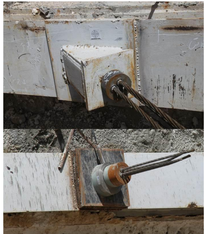
Fig. 18. ELC-30S Loadcell mounted on the anchor below to monitor the changes in the anchor pre-stressing load. Another anchor without a load cell is shown (above) for comparison.
