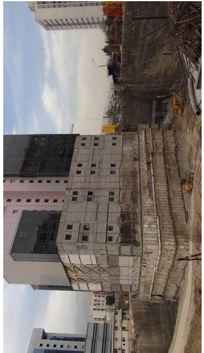
Fig. 15. A panorama view of the tower and the retaining system. In this image, all 4 levels of wailing have been installed.
