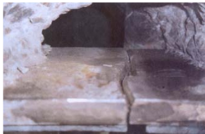
Fig 2. Crack in the top flange of a girder
