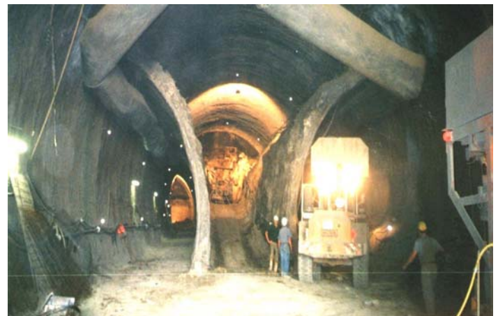
Figure 17. Side wall drift, picture from site
