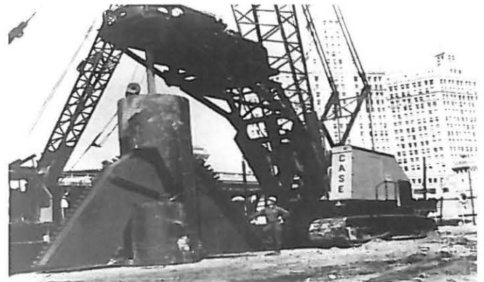
Fig. 17. Early Crane Attachment with First 7 ft. belling bucket capable of cutting a maximum 21'-0" diameter bell. (Circa 1963)
