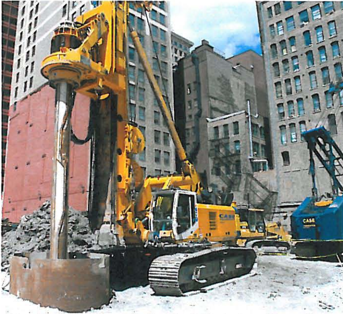
Fig. 32. Large Bauer hydraulic drill rig installing polymer slurry displacement caisson at Roosevelt University. (2010)
