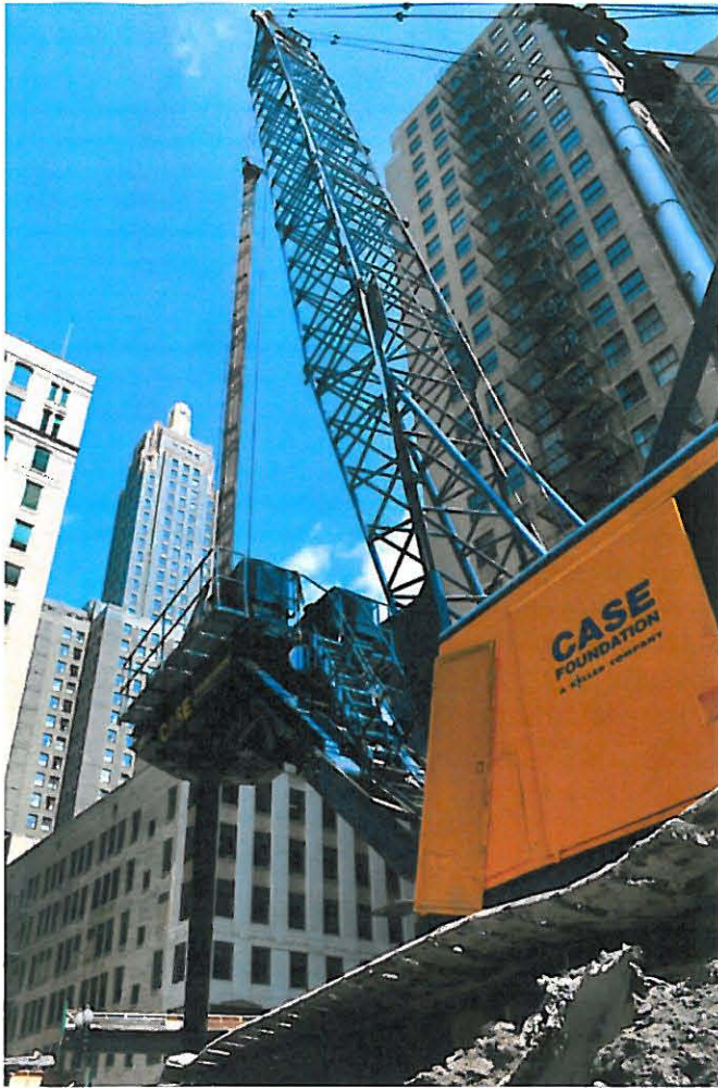
Fig. 23. Modern twin engine crane attachment
