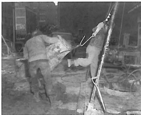
Fig. 10. Dumping well bucket of excavated material. Note air tugger (winch) and Tripod.
