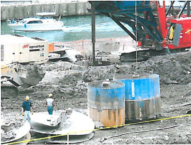
Fig. 29. 90" and 114" Hole Openers with calyx baskets in place above the canisters - Trump International Tower. (2005)
