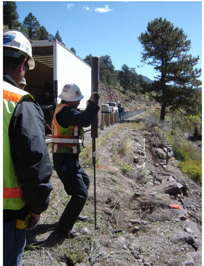
Fig. 14. “Jam” rod being driven just behind settlement zone at the top of the wall. This method of injection rod placement was fast, did not impact wall stability, and was sufficiently tight to inhibit resin from traveling up the outside of the rod.
