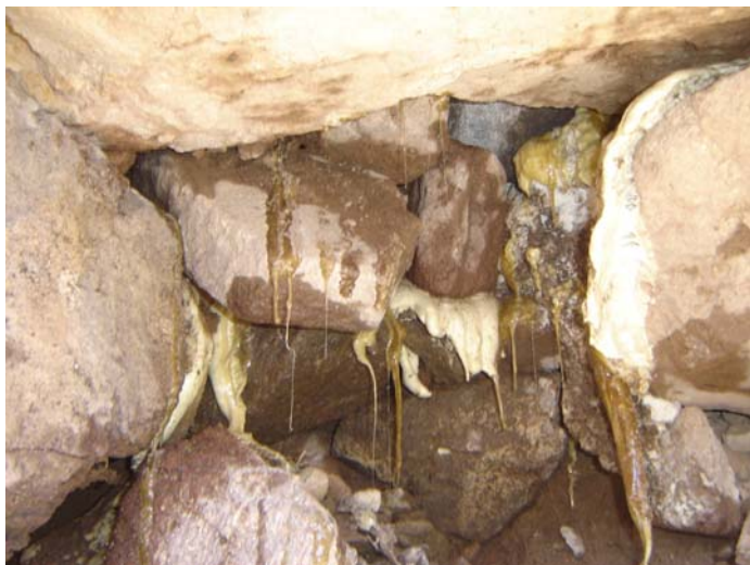
Fig. 16. Photo of interior of wall showing some void space is filled with foamed PUR, whereas most of the wall voids are coated with non-foamed resin.
