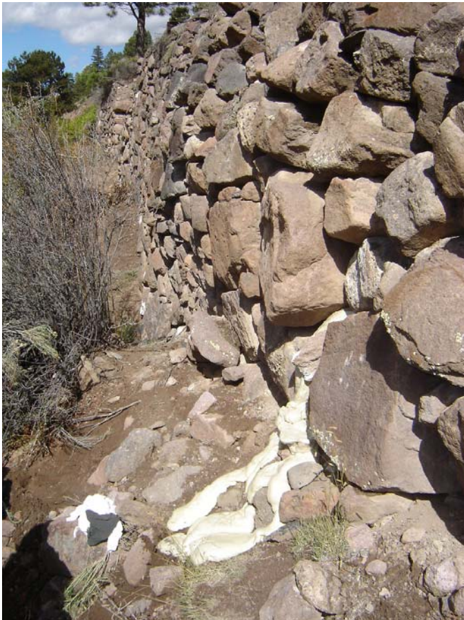
Fig. 13. Foamed PUR pouring from the wall toe during injection. Wet weather during the preceding days resulted in a foamed product until the wall dried days later.
