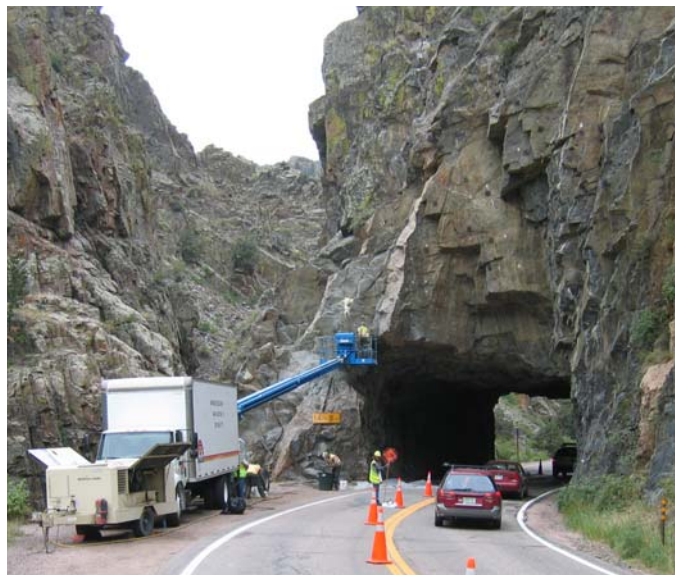
Fig. 2. PUR injection at the west portal of the Poudre Canyon Tunnel, along the Cache La Poudre River on SH 14.
