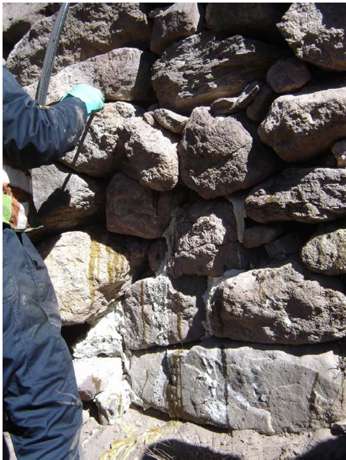
Fig. 15. PUR overrun experienced during face injection.
