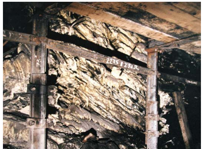
Fig. 5. PUR injected into coal mine roof and rib to stabilize failing ground conditions (note small-diameter injection rod extending from corner of opening).
