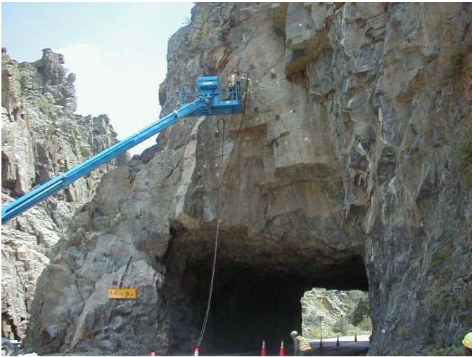
Fig. 6. PUR injection work in the bolted section above the western tunnel portal.
