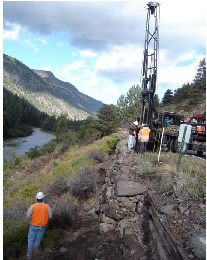
Fig.3 Drilling prior to PUR injection behind a dry-laid stone masonry retaining wall along SH 149 west of South Fork, CO.
