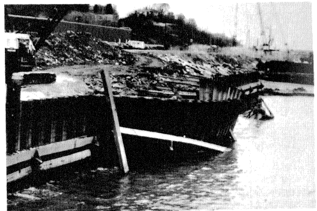
Fig. 5. Photographs of Bulkhead After Failure
