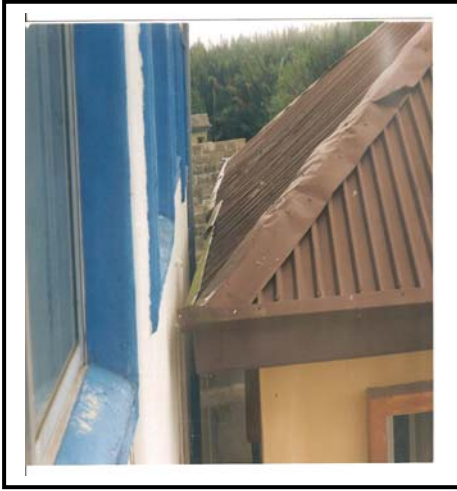
Fig. 7c. A view of the house leaning on an adjacent building
