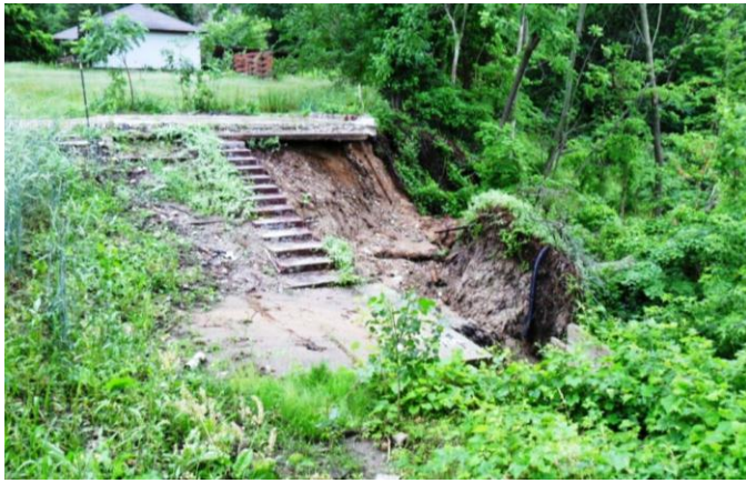
Fig. 6. Translational Slide - Condemned Residence (2011)
