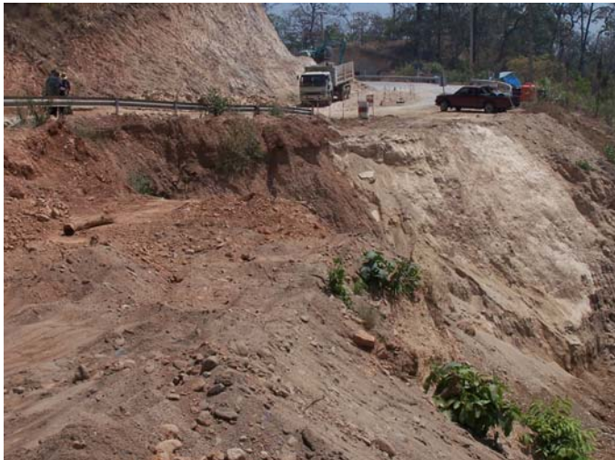
Figure 2: Site with Sloped Embankment Failure
