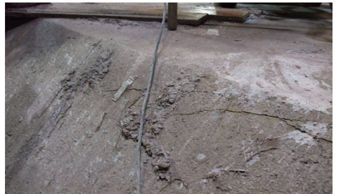
Fig. 15 – Cracking to tank base slab in vicinity of the sump.
