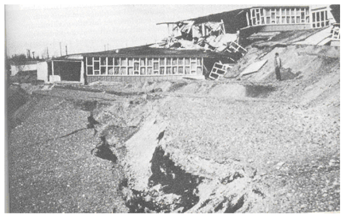
Fig. 5. School building that collapsed as a result of a landslide at Government Hill, Anchorage, as a result of the Alaska, 1964 earthquake (Bolt, 1978).
