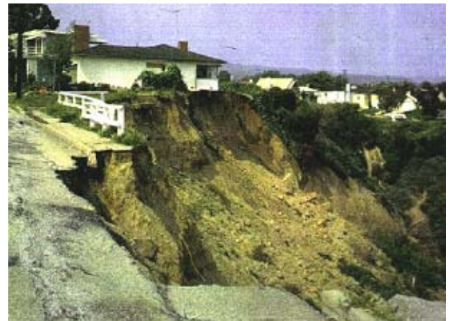
Fig. 12. Structure affected by a slide as a result of heavy rain in 1969 at Palisades –Potrero Canyon - Friends Street, California ( http:// geology.wr.usgs.gov/wgmt/elnino/scampen/examples.html , 2006)
