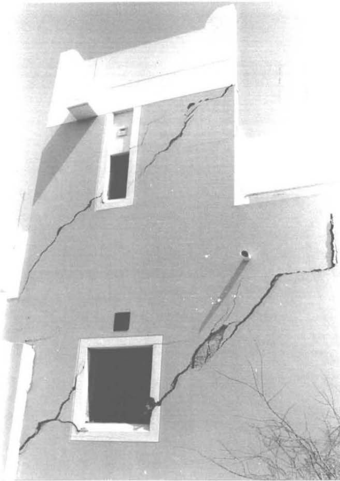
Fig. 6 Back elevation of house number 18 showing extensive damage to the wall.
