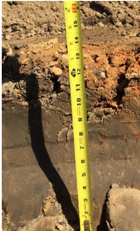
Figure 17: Depth of Poorly Compacted Soil
