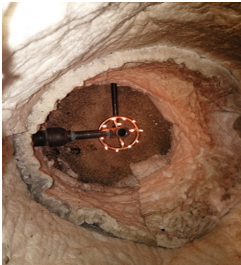
Figure 2.7. Top view of combustion chamber showing insulation, ring burner and syngas outlet opening
