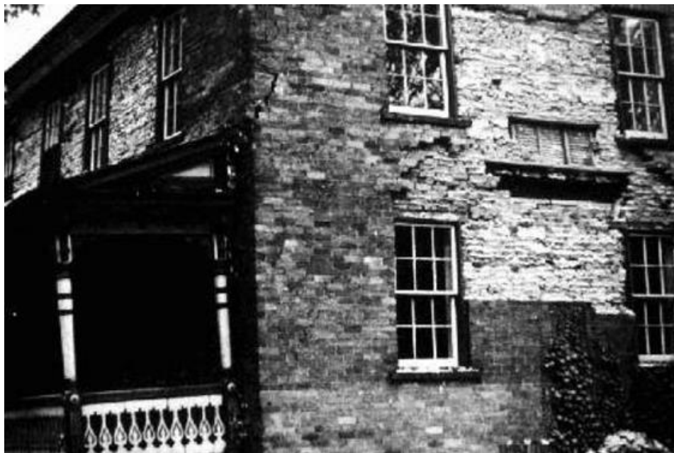
Figure 3. Photograph of damage on the south and west sides of a house in Cornwall. Cracks can be seen in the corners, as well as collapse of the outer veneer walls (Berkey, 1945).
