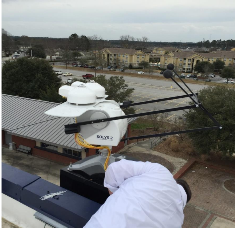
Figure 11: Kipp & Zonen SOLYS 2 Sun Tracker installation at Georgia Southern University Paulson Stadium
