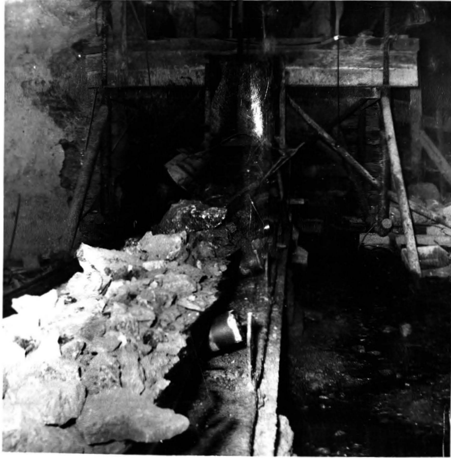
Fig. 4 Feeding fluorspar ore onto a 30 inch belt conveyor. Dump trucks discharge onto a portable 15-ton steel hopper, which is covered with a grizzly with 8-inch bar spacing. The slope to the top of the hopper is built from waste rock. The hopper can be dragged ahead when the belt is extended.
