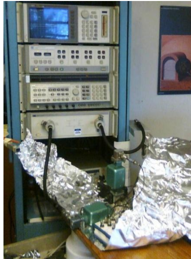
Figure 5.24. Metal foil for ground-noise removal.
