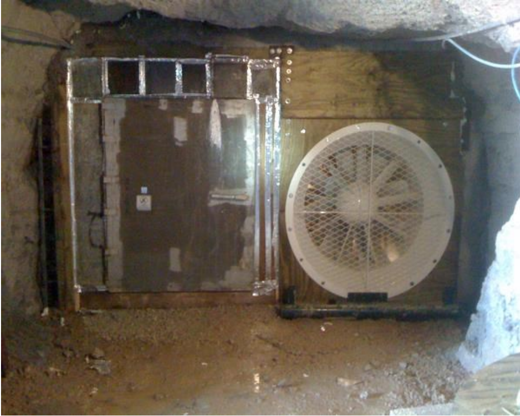
Figure 3.11 Booster fan bulkhead- rear view
