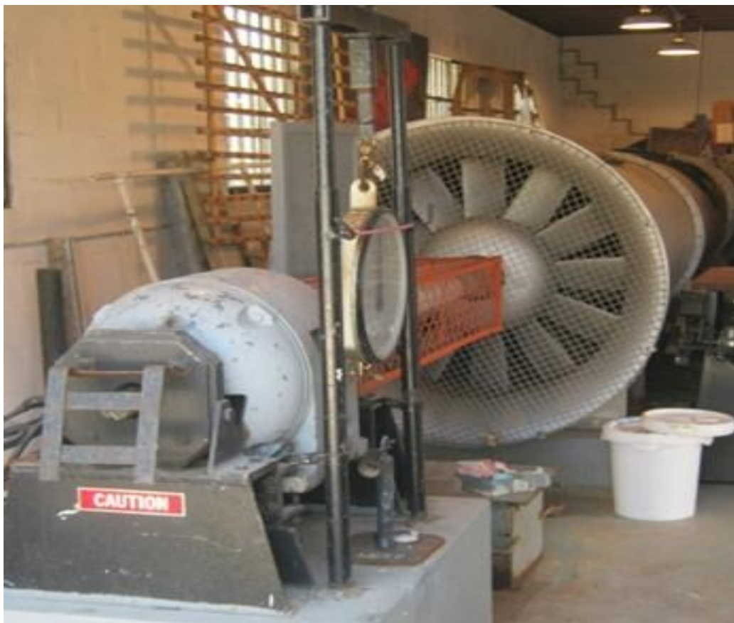
Figure 3.4 Missouri S&T surface main fan
