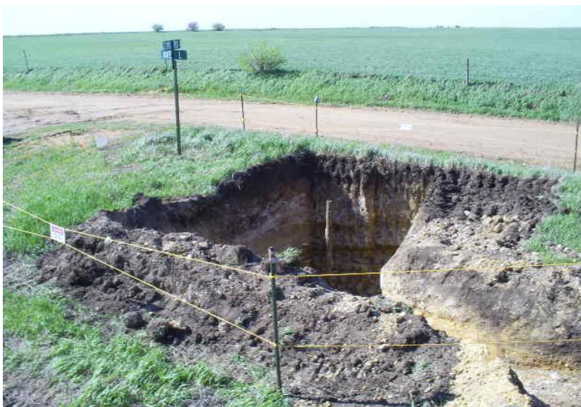
Figure 8 Exposed abandoned well casing located 0.6 meters below ground level. View Southwest
