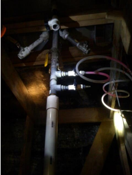
Figure 12. Air manifold for the pressure/volume test.
