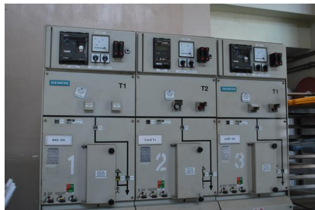
High Voltage Switchboard Training in IVE (Haking Wong)
