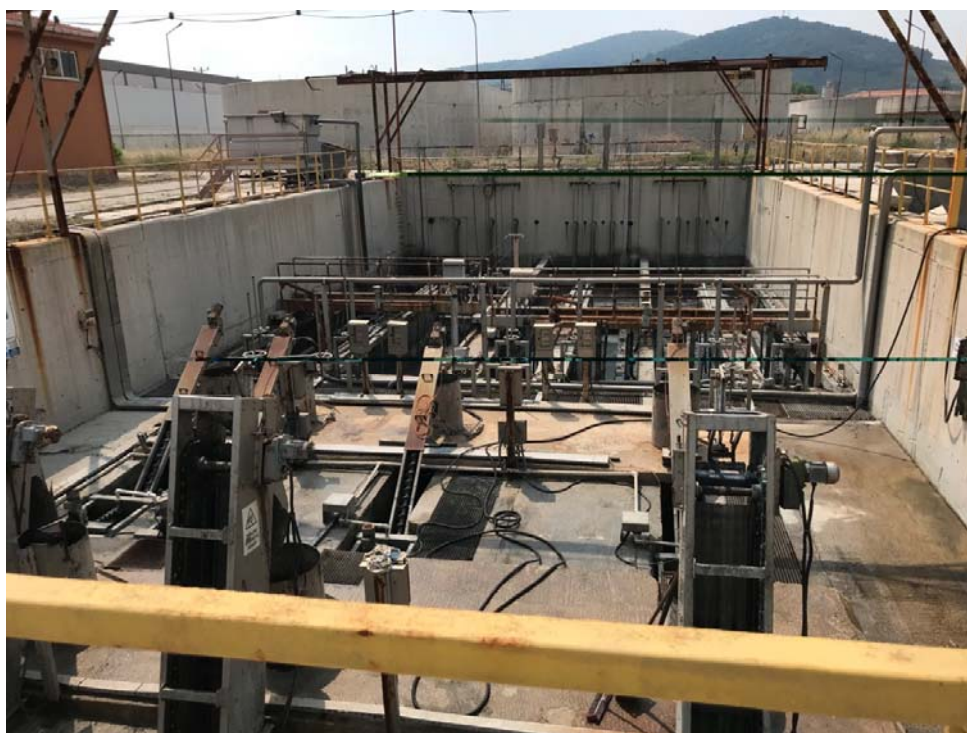
Figure 2. Entree Unit in CETP
