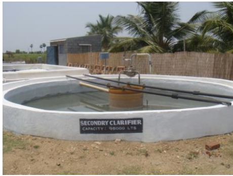
(g) Secondary Clarifier
