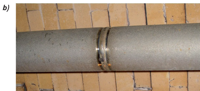
Fig. 4 - Edge preparation for butt welding of tube pieces (a), welded joint (b).
