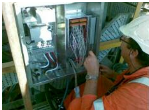
FIG. 4 Field cables and termination in an on-line instrument at a refinery.
