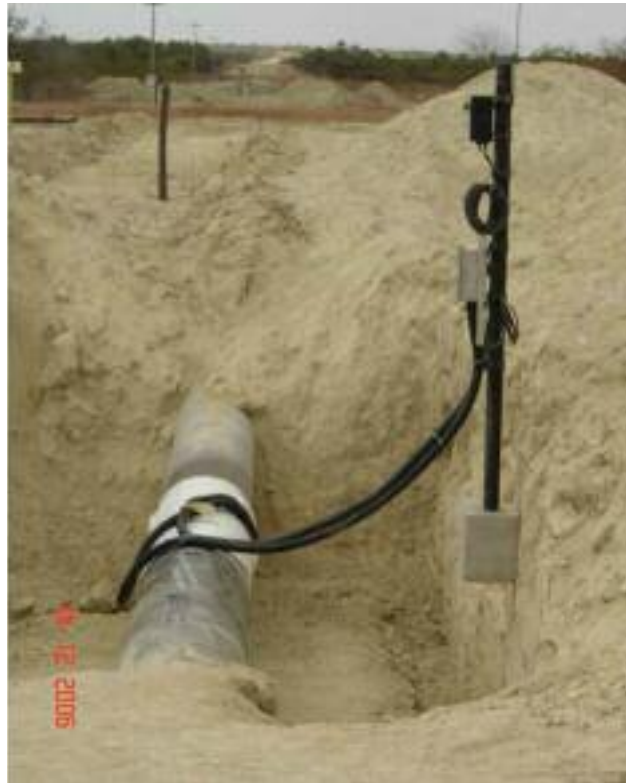
FIG. 3 An off-line electric field signature system on an underground pipeline in Brazil. Cable from the instrumented pipe section is pulled to junction boxes for connection with the portable instrument for data collection. After installation, the pipe will be covered by soil, and only the connection post will remain visible.
