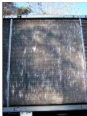
Uncoated fouled and corroded units.
