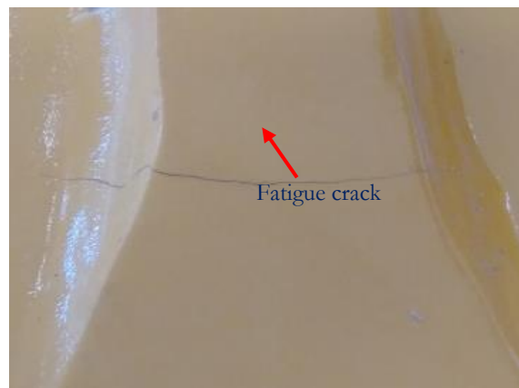
Figure 5: Fatigue failures on moving arm of No.2 excavator, which is the same as failure position of No.1 excavator
