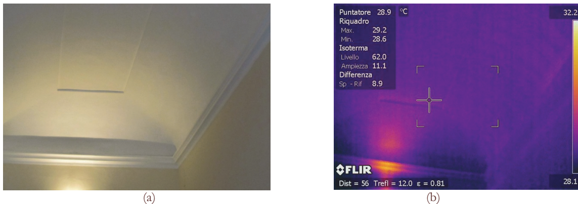
Figure 6: Room 48: (a) view and (b) thermographic image of the intrados of the vault.
