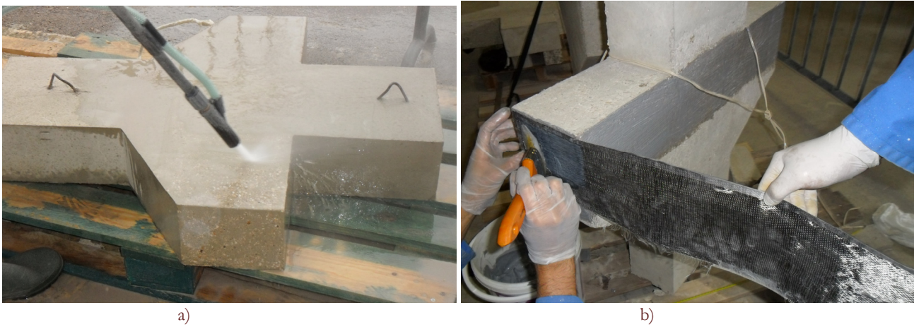
Figure 2: Details of bonding system of: a) Sandblasting of corbels and b) Application of carbon fiber on concrete surface by wrapping.
