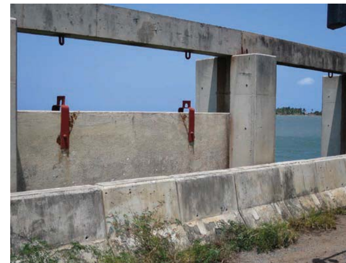
Volta sluice gate (Photo: Katharine Vincent)
