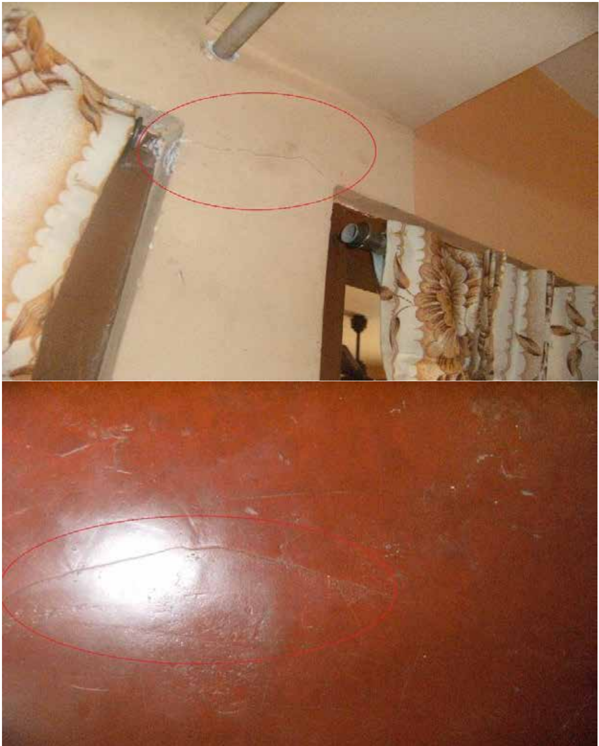
Figure 10: Cracks and Seepages
