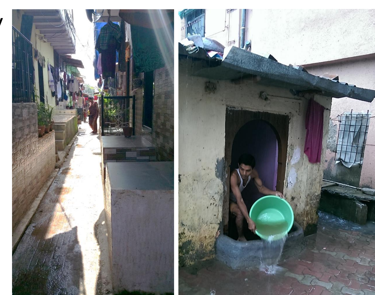
Structural modifications such as elevating the plinth and cement bunds around doorways are structural coping measures. Source: Photograph by author, 2015
