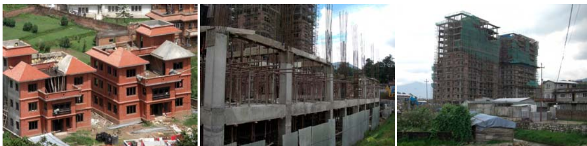
fig 39 – Development on project scale is growing. Multi-storey buildings become more popular in Kathmandu. (Pictures Tjerk Reijenga)
