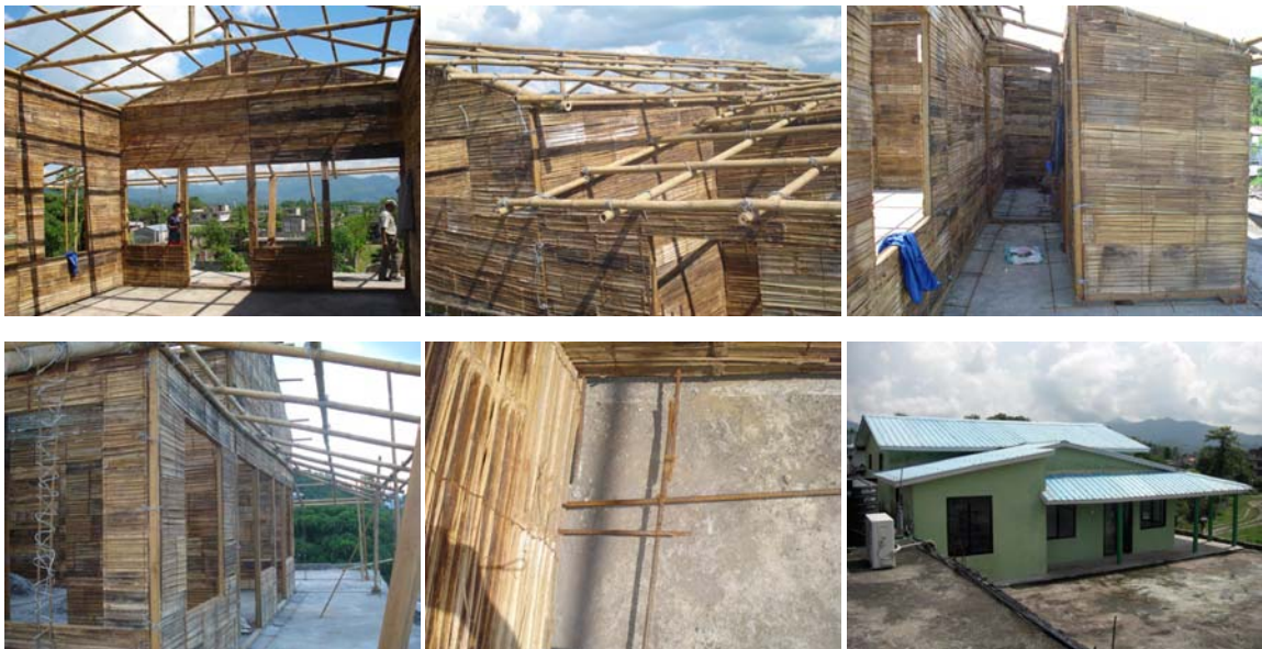
fig 37 – Bamboo house in Lekhnath. Built as an extension on the roof of a concrete building. (Pictures Tjerk Reijenga)
