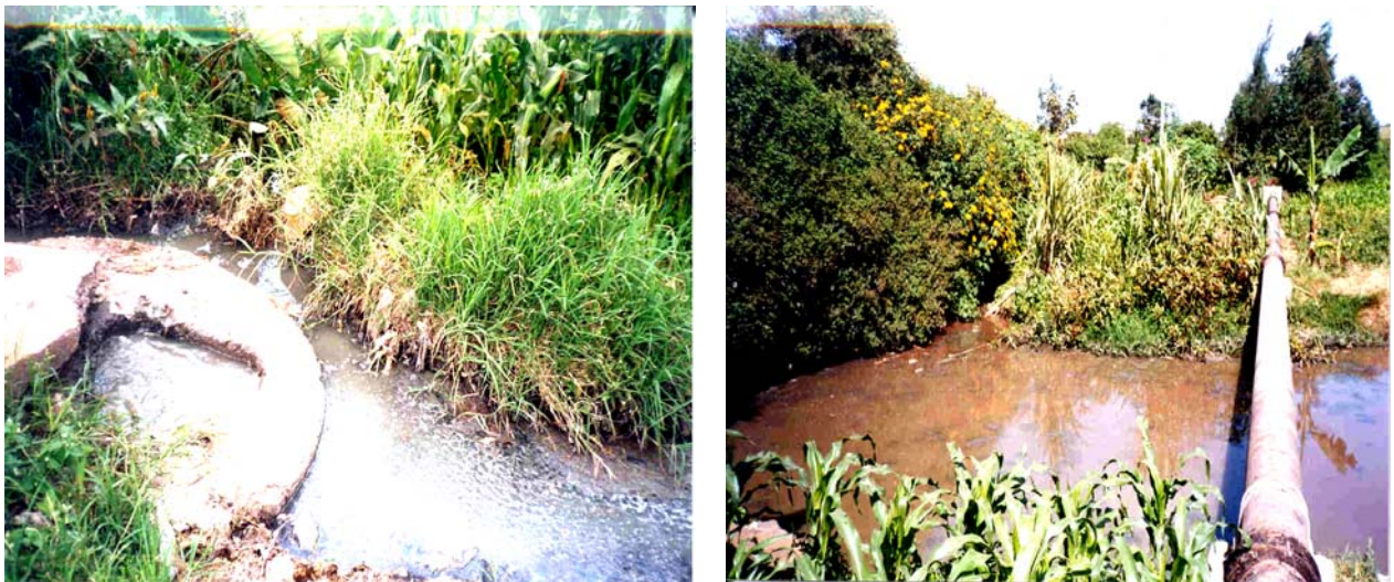
Figure 10: Blocked manhole and a sewer line crossing through Maili Saba.
