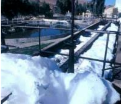
A water purification plant in Amman. (IDRC Photo: Peter Bennett)
