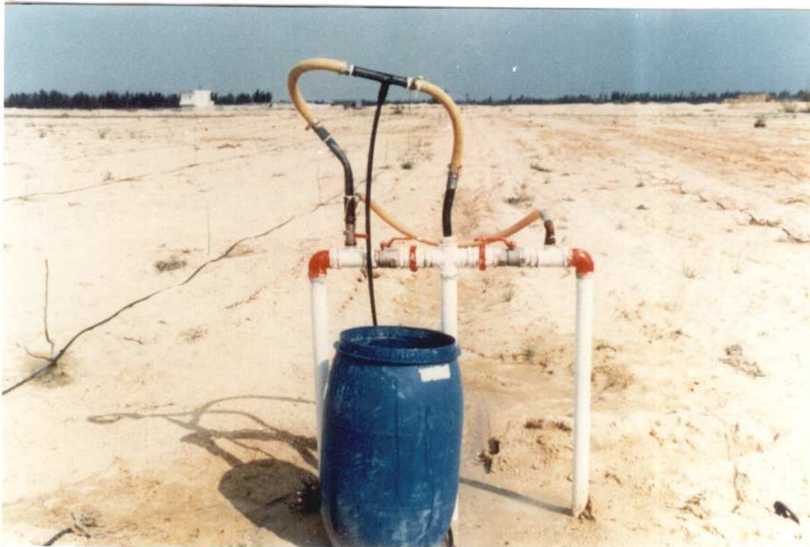
Fig. 5.9 Venturi Fertilizer injector installation
