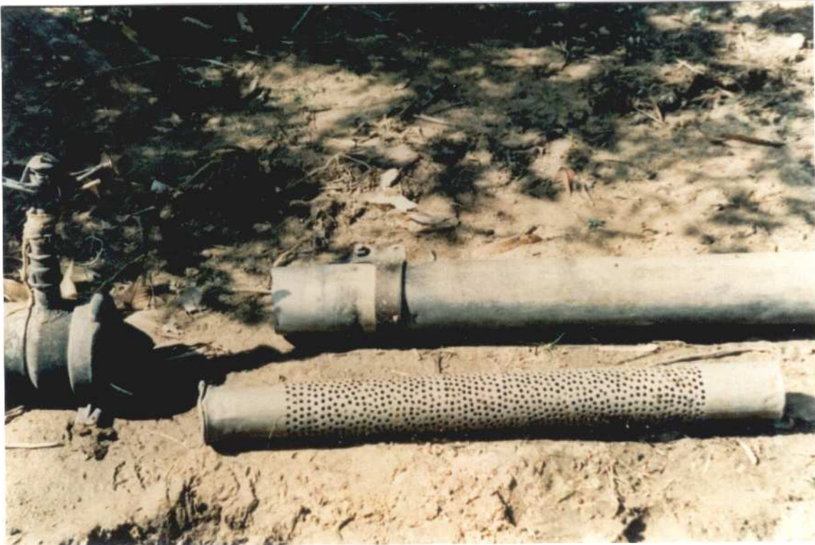
Fig. 5.4 : Making the Screen lip by Pounding on the Pipe edge to bend it into the form of a lip
