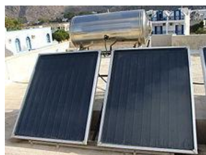
Flat plate thermal system for water heating deployed on a flat roof.
