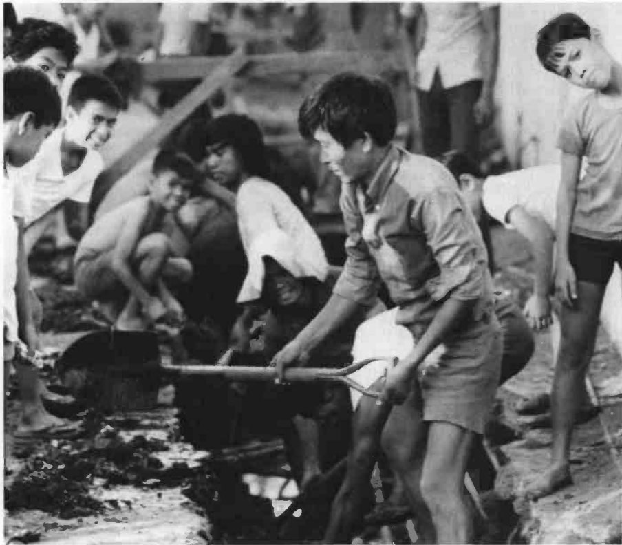
Digging drainage canals using the mutual-aid approach in the Tondo project, Philippines — an effective method of reducing construction costs.
