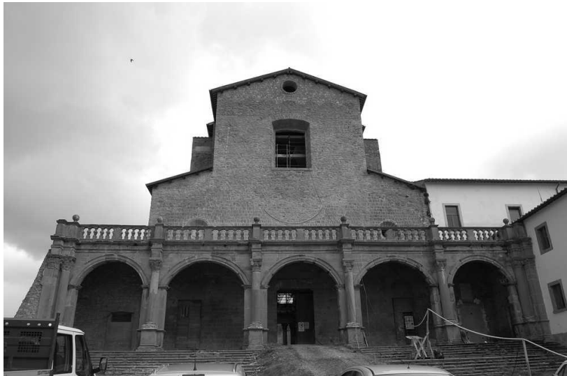
Fig. 6 The front of the church of St. Mary in Gradi during reconstruction [6]
