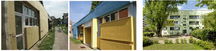
Fig. 1 Facility “Ivancica” during execution works on thermo-insulation and appearance after project completion (left), Nido Piccolo Day Care Centre (right)
