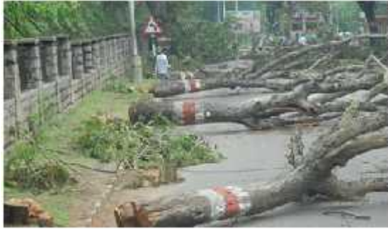
Plate 22. Cutting avenue trees for road widening in Krishnaraja Sagar Road - close to the Railway Station
