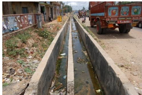
Plate 2: Unmaintained open drainage used to throw the waste in major city road
